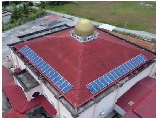
EPCC of solar PV system for a Surau under FiT programme
