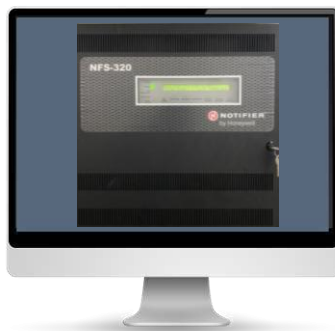
Fire alarm control panel
